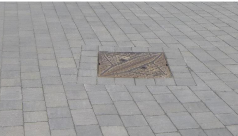
Figure U2: Awkwardly aligned access cover is made apparent through use of setts
