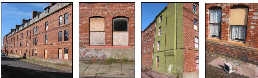
Egerton Buildings (middle and far left) have many windows boarded up. The seaward face of the building (middle right) is in poor condition and there is evidence of continued vandalism and poor quality repairs (far right)
