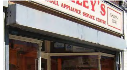
Bulky and unsightly roller shutter housing obscures the top of the shopfront
