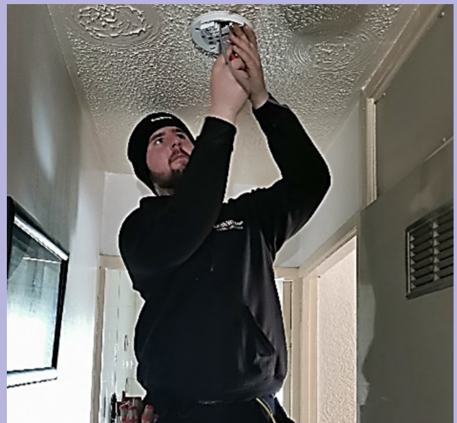
Dylan from Keith Wilson Electrical fits a carbon monoxide alarm in a tenants' home
