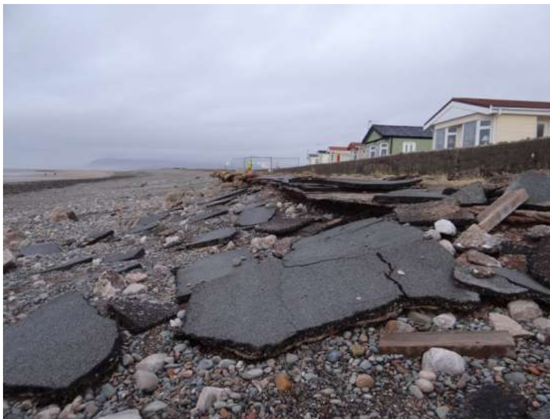
Erosion at West Shore Park, Walney Island, 2013
